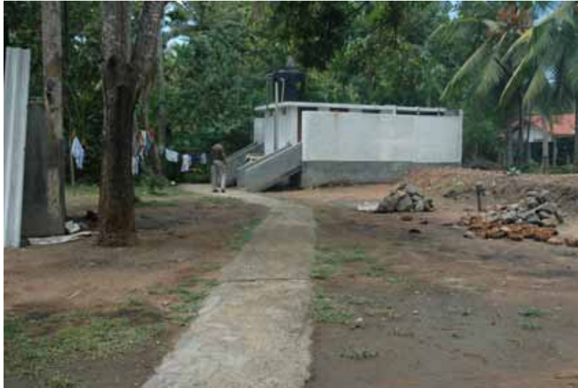
NEW TOILETS WITH NEW PATH THAT IS ESSENTIAL IN MONSOON AND ALSO REDUCES CHANCES OF SNAKE BITES IN THE BLIND CHILDREN.
